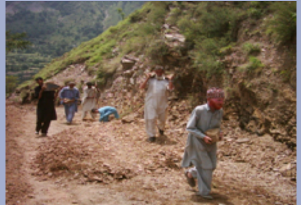
Widening of village link-road at Pekho Nakar Union Council Abbottabad district (NWFP) in the context of the Livelihoods Rehabilitation Strategy of ERRA supported by FAO.
